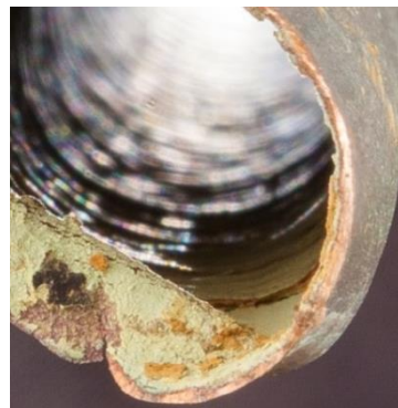
Figure 3. West Saint John Copper Pipe Close-up
